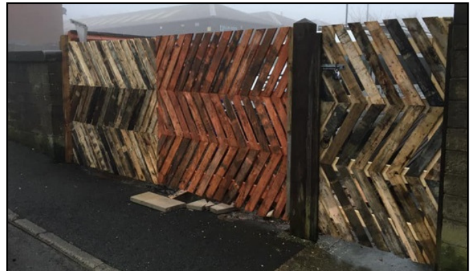
Sessional worker Bernard Tighe did a fantastic job rebuilding the gates at the VIC Centre which were damaged by storms Ciara and Dennis.
